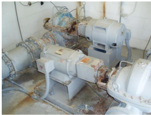
Older equipment in poor condition may have a greater electrical failure potential.
